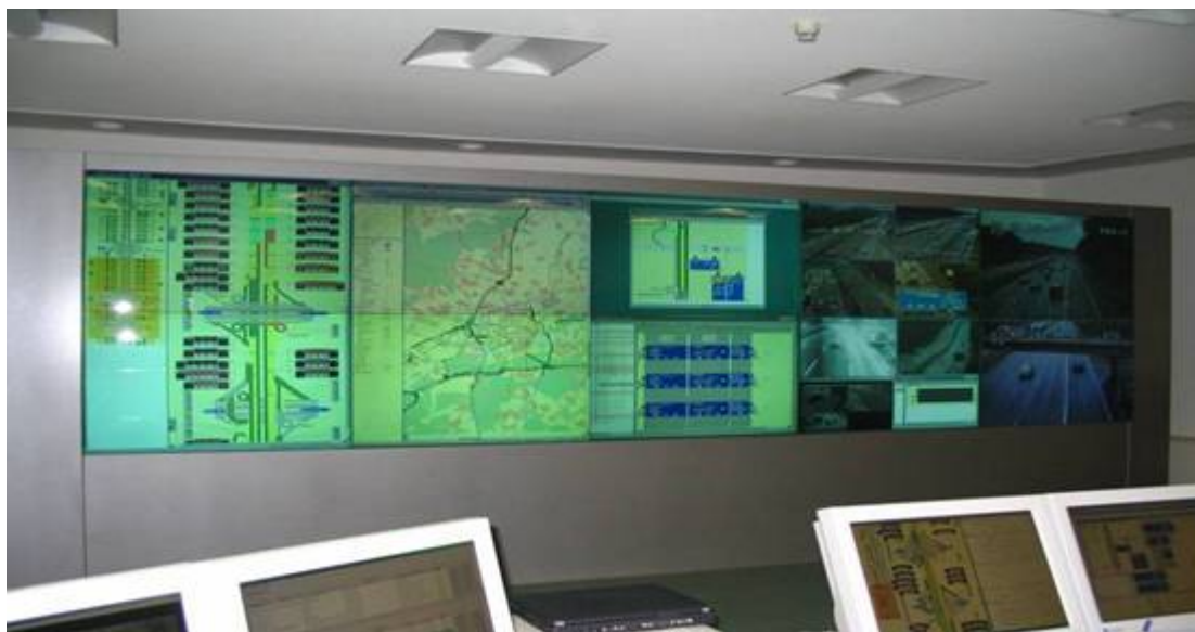
Figure 21: Control room in Germany, showing map-based systems
