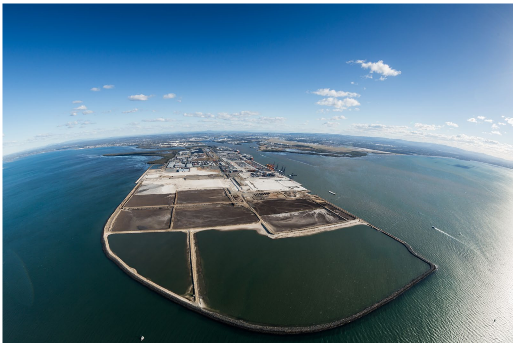
New container terminal under construction, Photo courtesy of Port of Brisbane Pty Ltd.
